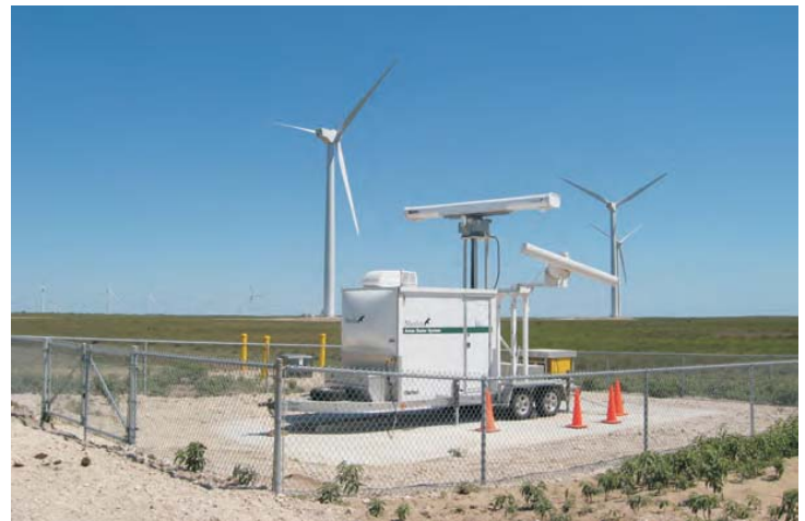
ABOVE: MERLIN SCADA installation at the Iberdrola Penascal wind farm in Texas, USA (operating since 2009)
