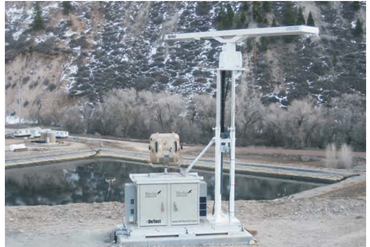
Skid-mounted single MERLIN detect & deter system for small gas processing facility waste pond resident & migratory bird control (Colorado USA).
