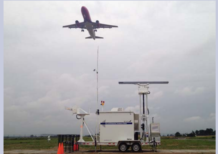
ABOVE: MERLIN Aircraft Birdstrike Avoidance Radar system installation at the Warsaw, Poland airport.
